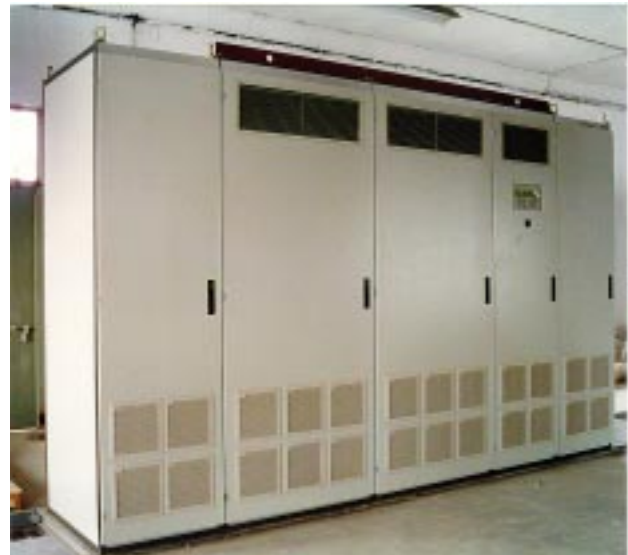
AC drive panel
